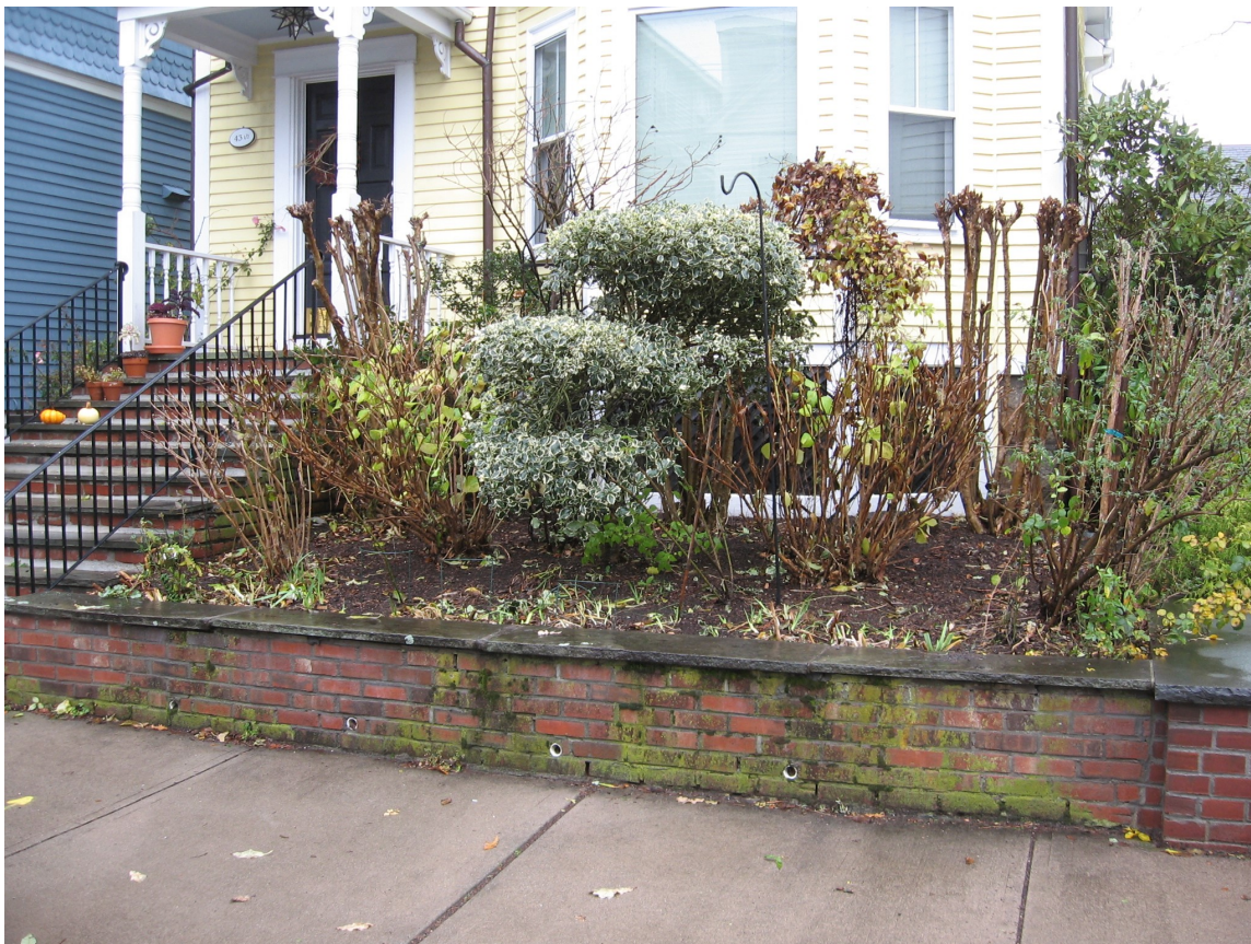
The dwelling at 431/2 Elm Street displays a planter wall and landscaping which provide some resistance to flooding.
