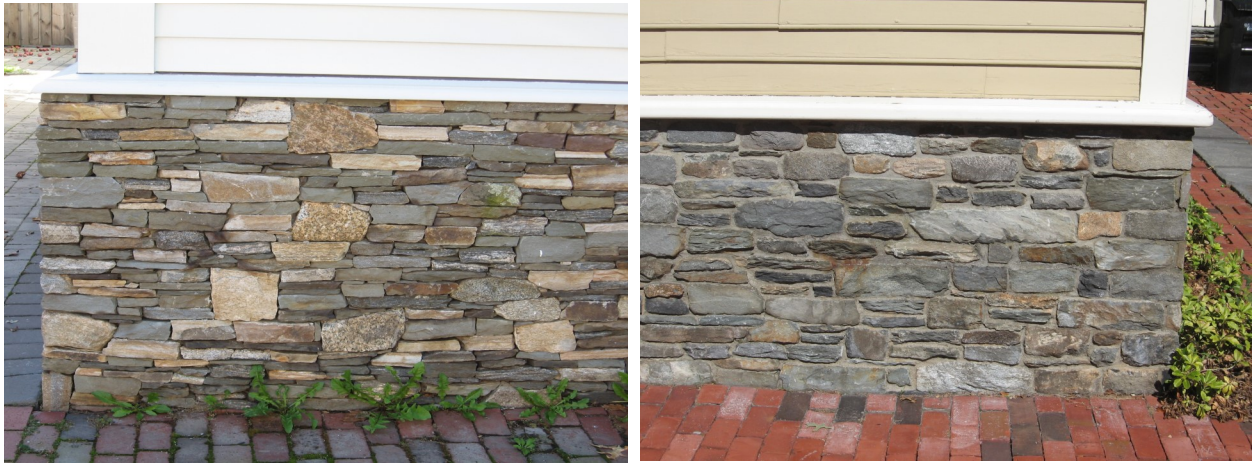
The rebuilt foundations at 62 Bridge Street (left) and 31 Walnut Street (right) reused existing stone and were designed to complement the original designs.
