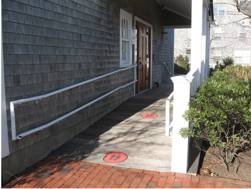
Some low-elevation projects may be able to utilize ADA ramps on the primary façade. Such ramps should be in traditional designs and screened (Nantucket, Massachusetts).
