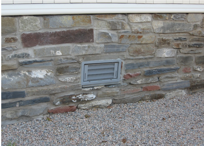
Example of a standard size flood vent and appropriate location one-foot above grade at 74 Bridge Street.
