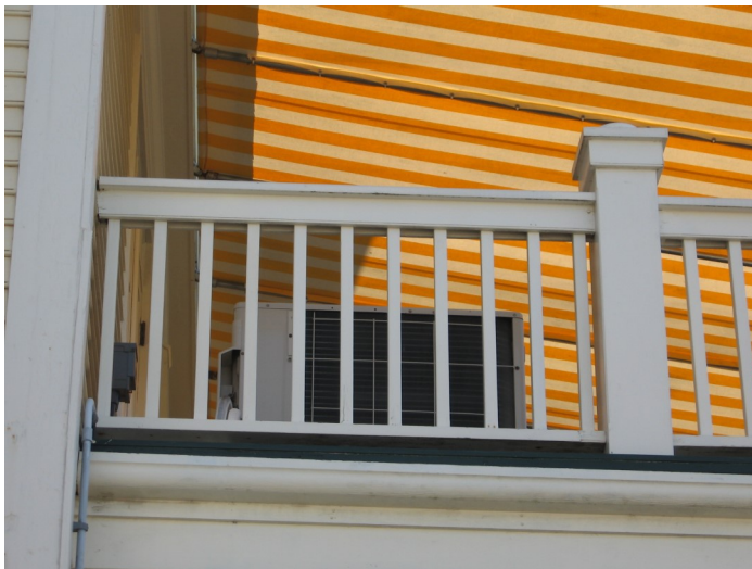
Appropriately sited and screened HVAC unit on the second floor rear porch at 62 Washington Street.
