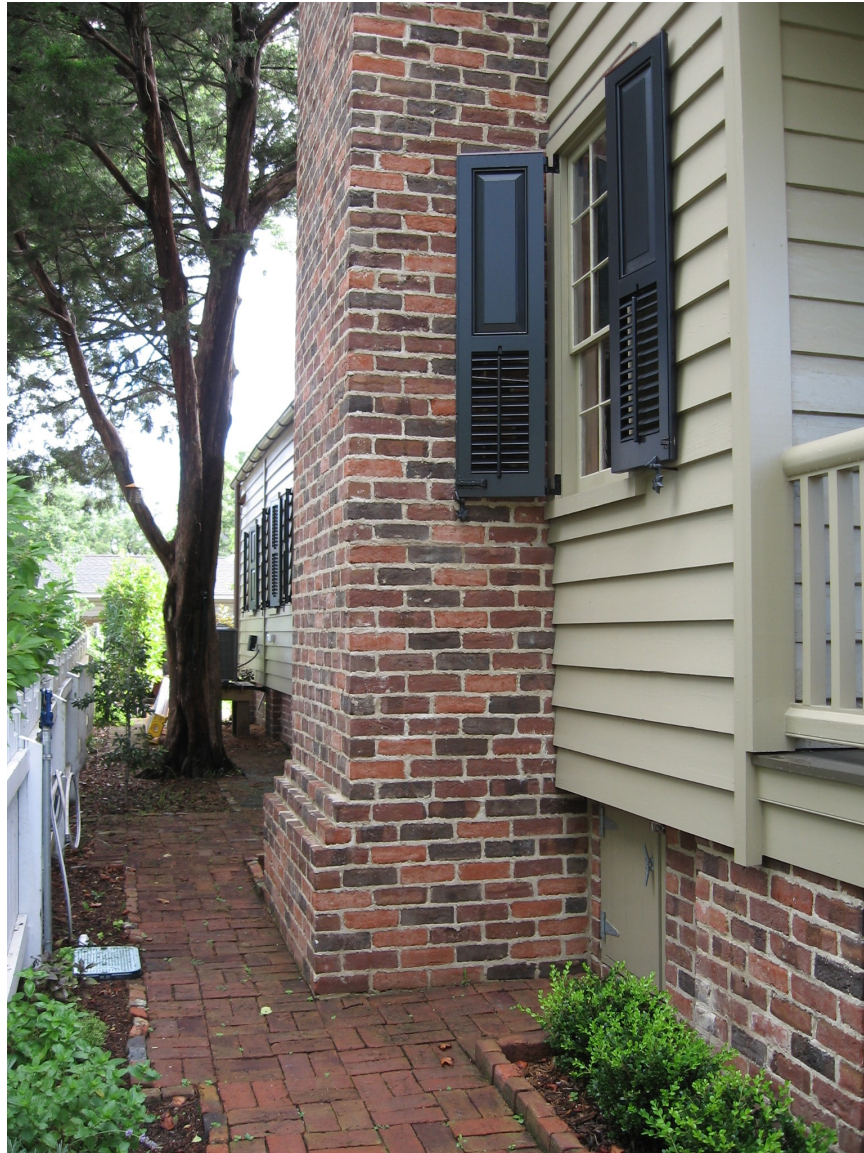
The elevation of this dwelling included rebuilding the base of the chimney with brick and mortar to match the original (Beaufort, South Carolina).
