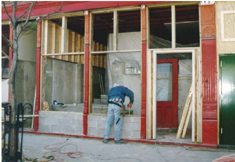
Another strategy for dry proofing commercial buildings is to harden the storefront and raise the interior first floor level. In this approach the frame storefront bulkheads are replaced with concrete and a parged surface (above).
